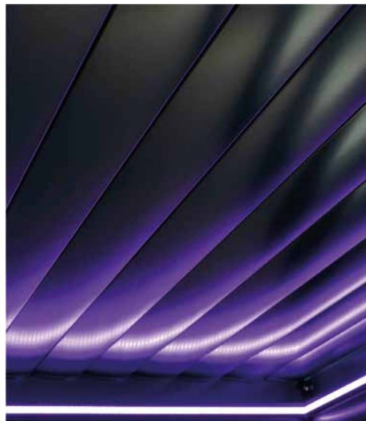
• Roof louvers in closed position
